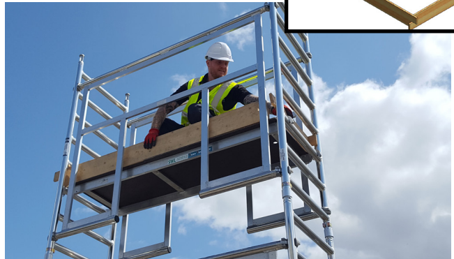
14. Fit toeboard lengths and ends as shown by slotting the wood into the designated area on the clip.
